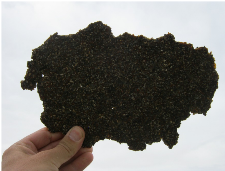
Figure 4-8 Polymer overlay deterioration.
