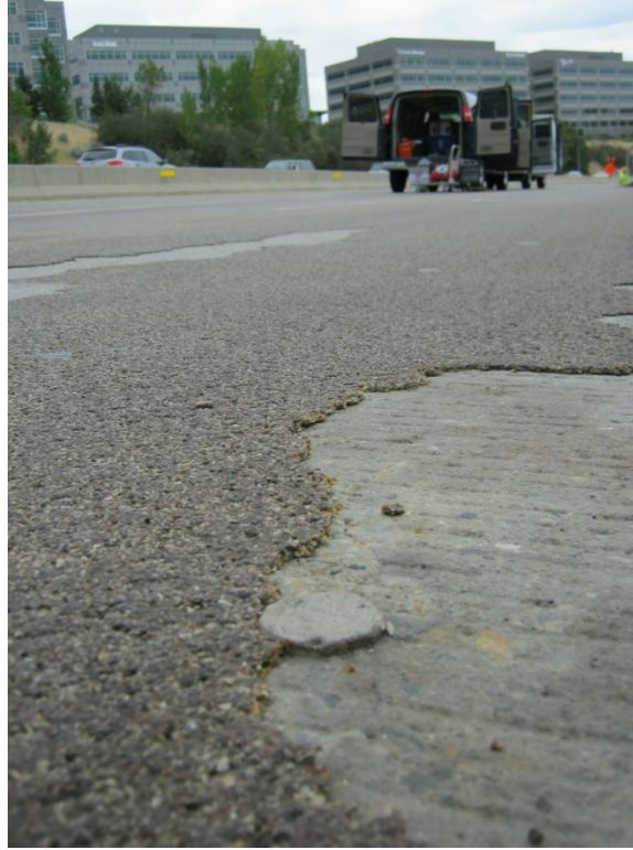
Figure 2-37 Failing polymer overlay.
