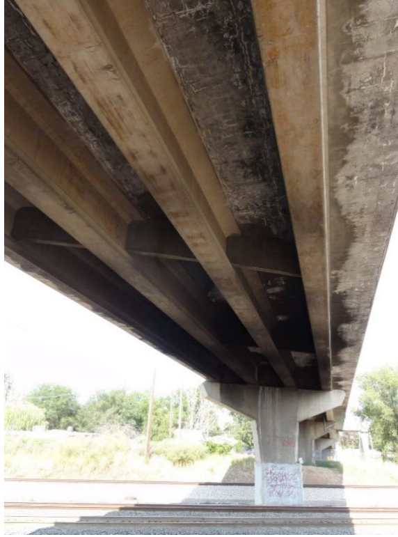
Figure 4-7 Significant cracking and efflorescence on the underside of a bridge deck.
